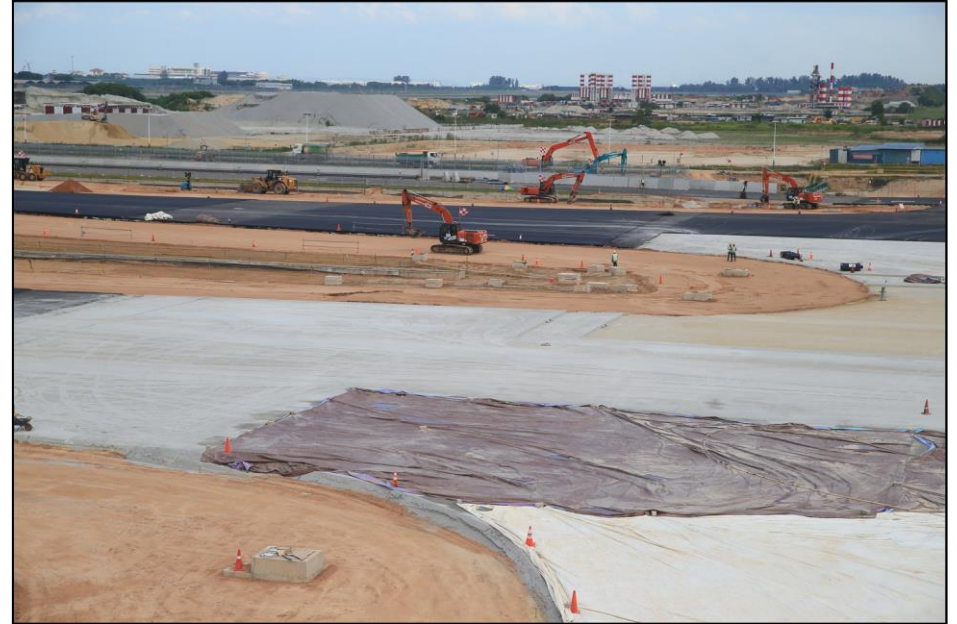
10G CTB with no pre-cracking
